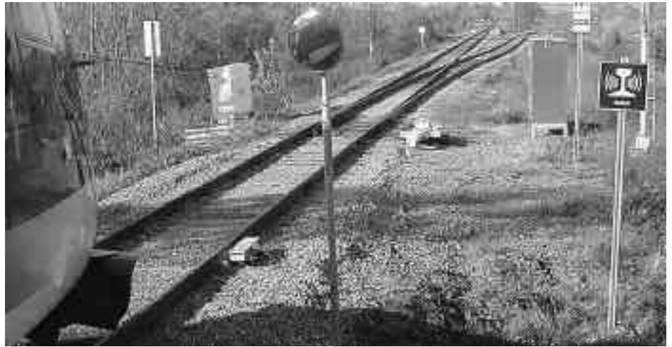
Indusi magnet at north end of Greenboro station protects diverging line to Walkley Yard — Indusi magnet is next to track, with sign placed to remind operator.
