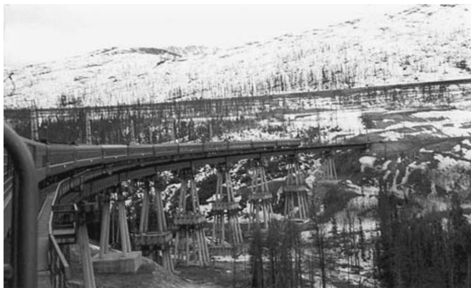
Chertov bridge on the BAM. Piers are concrete circular columns resting on massive footings. Middle pier footings sit on lower piers made of more circular columns.
