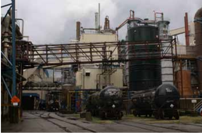
Photo 3: As a prototype, this maze of pipes and scaffolding is rather intimidating to a railroad modeller. Nevertheless, one need only replicate a sense of this complexity in order to render a credible model.
